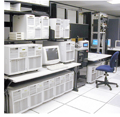
Network Operations Center
