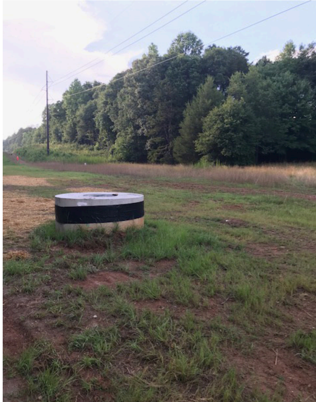
ReWa Sewer Trunk Line Easement in Five Forks.
