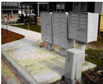
CORRECT – NOTE HOW MUCH CONCRETE WAS REQUIRED IN ORDER TO MEET LOCAL CODES
