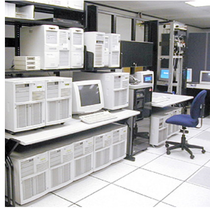
Greenville County Server Room
