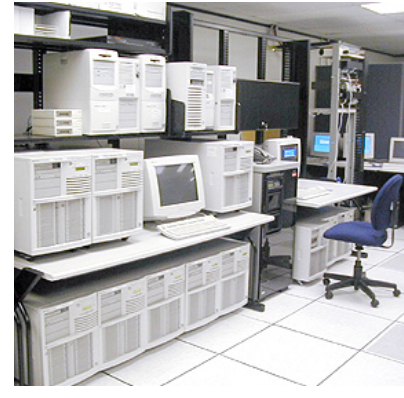
Network Operations Center
